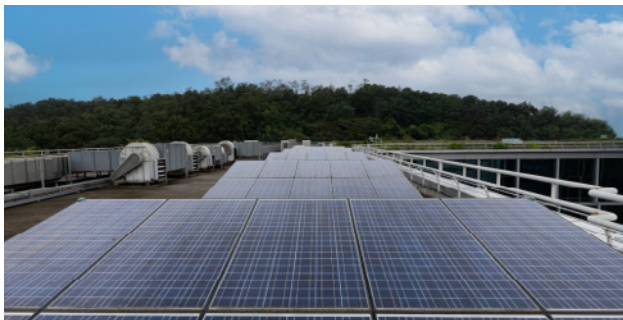
Solar Power System
