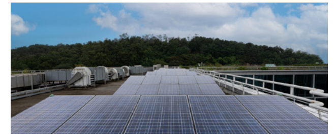
Solar panels at the Pangyo business site
